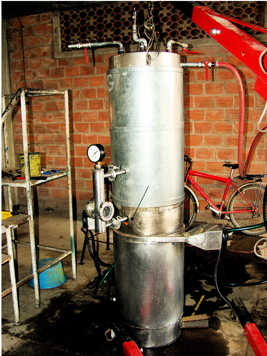
Photo 5: Gasifier/ boiler at work, no visible smoke on top, flame is clearly visible (arrow)
